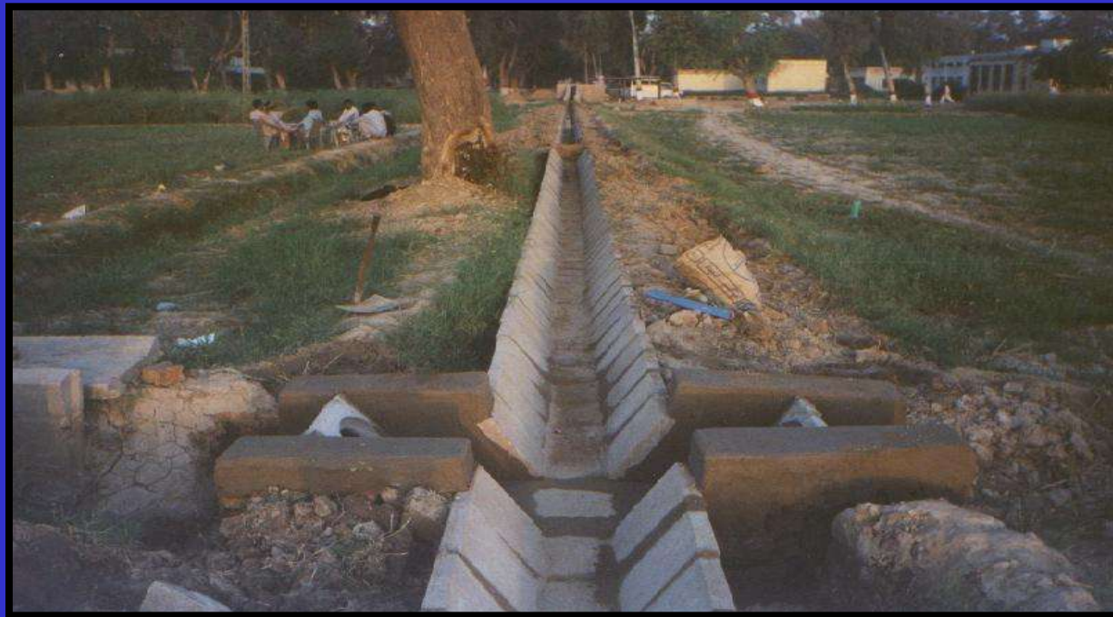
View of channel lined with Precast Lining Unit Developed by CWHR at Tandojam
