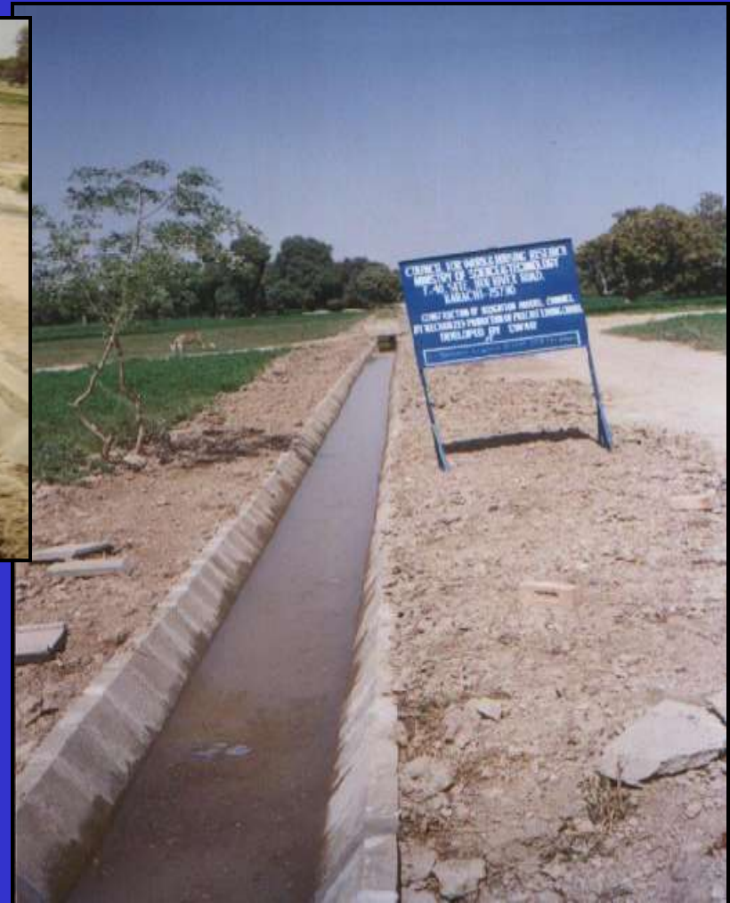
Model channel constructed at Horticulture Research Farm, Mirpurkhas, Sindh with precast lining units
