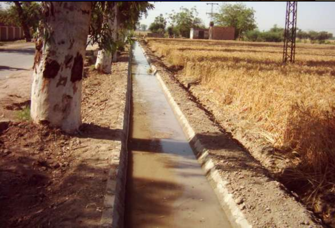
Model Channel constructed at Adaptive Research Farm Vehari, Punjab with Precast Lining Unit
