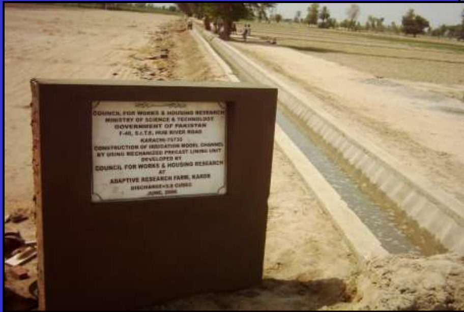
Model Channel constructed at Adaptive Research Farm, Karor, Liyyah, Punjab with Precast Lining Unit
