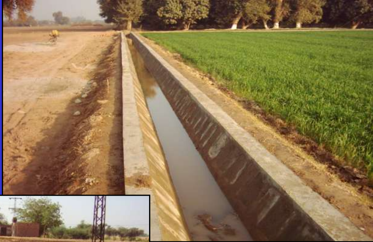
Model Channel constructed at Adaptive Research Farm Rahim Yar Khan, Punjab with Precast Lining Unit
